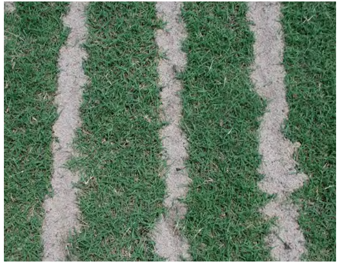
Sand-slit drain trenches backfilled with sand - Photo courtesy of Brad Fresenburg, Ph.D.
