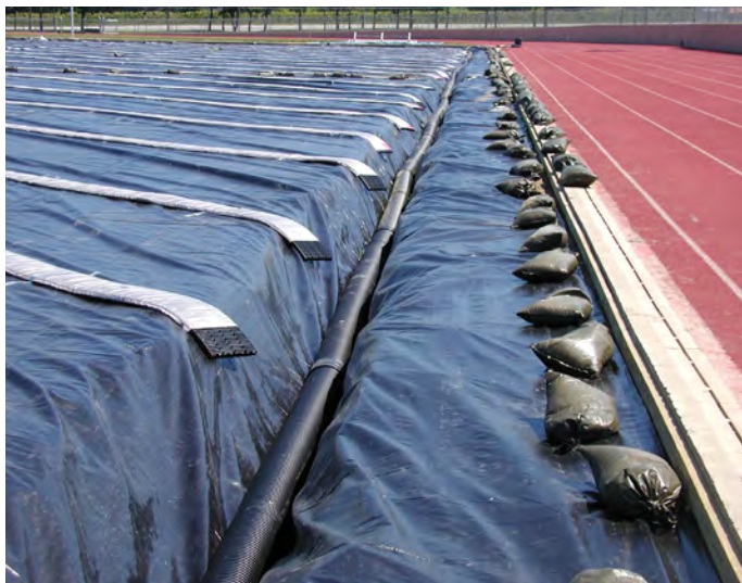
Strip drains to collector pipe - Photo courtesy of Brad Fresenburg, Ph.D.
