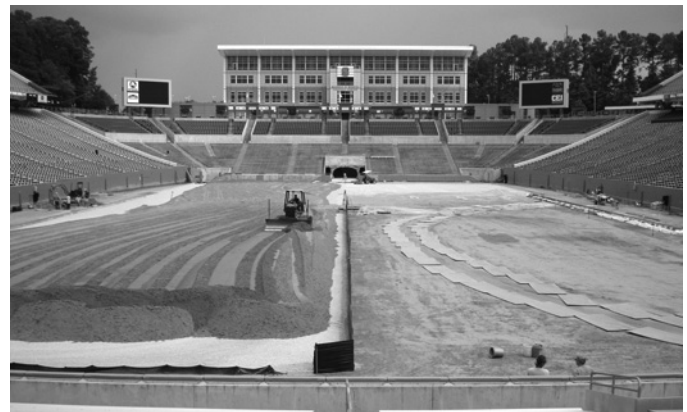
A smaller laser-guided dozer used to spread soil mix. Note use of silt fence and plywood to protect sub-surface layers.
