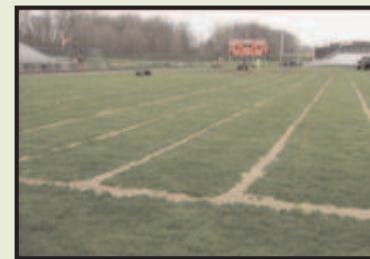
May 2007. Grand Blanc High School athletic field after the drain line installation process, Grand Blanc, Mich., Water Management Inc.,
