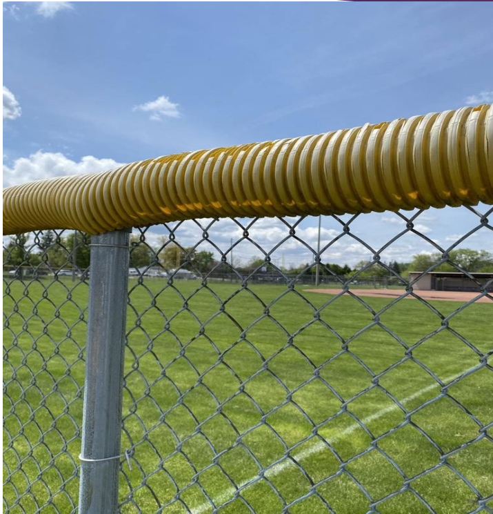
Eroded fence capping
